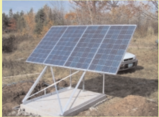
Stationary mounted panels can be adjustable, permitting the panels to face the sun as near to perpendicular as possible.
