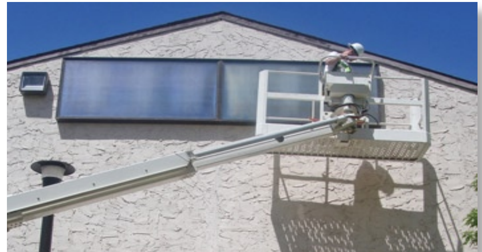
A solar hot air installation at the Little Earth Housing Development in Minneapolis.
